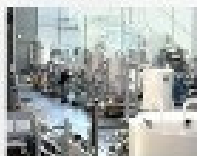
PUMP SKID SYSTEM
